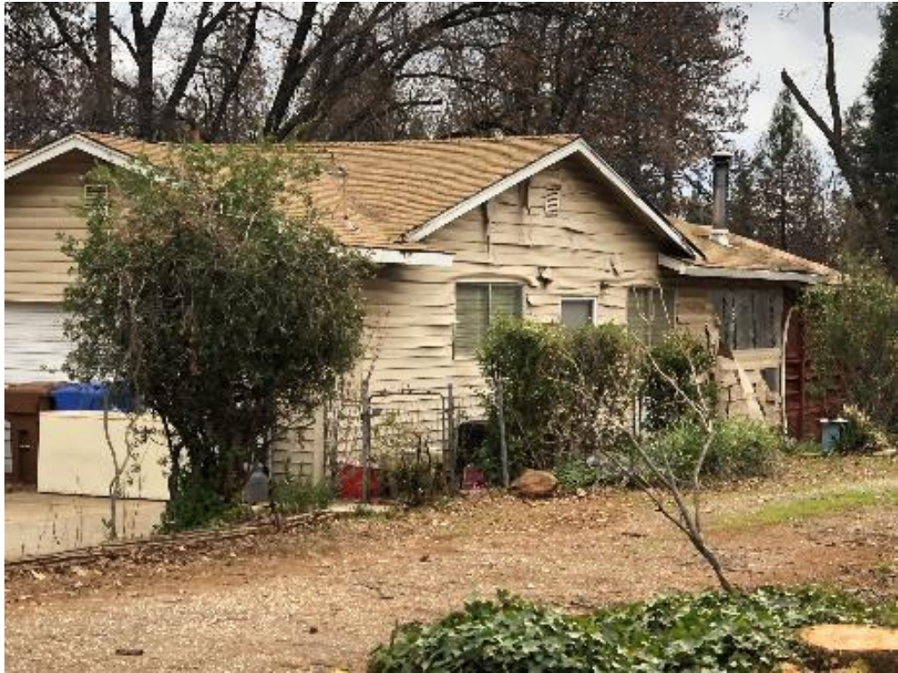
Figure 5: Example of Partially Damaged Structure following Wildfire
